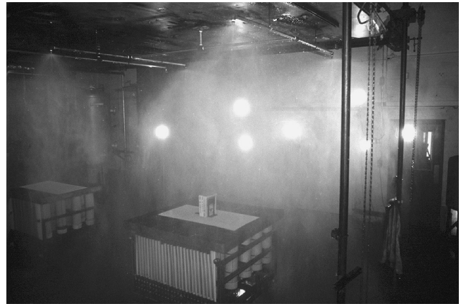
FIGURE F.3(b) Water Mist Discharge.
