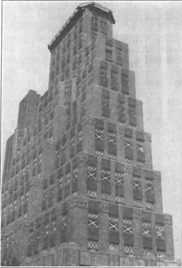
Scaffolding removed except small one at tower, which took fire.
