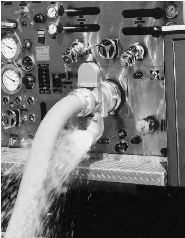
FIGURE D.5.4 Intake Gated Relief Valve.
